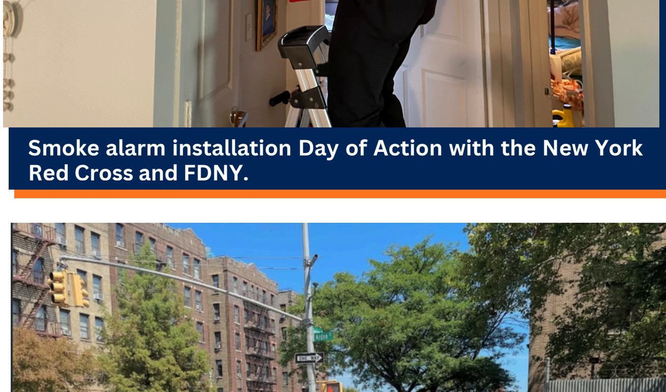
Smoke alarm installation Day of Action with the New York Red Cross and FDNY.
