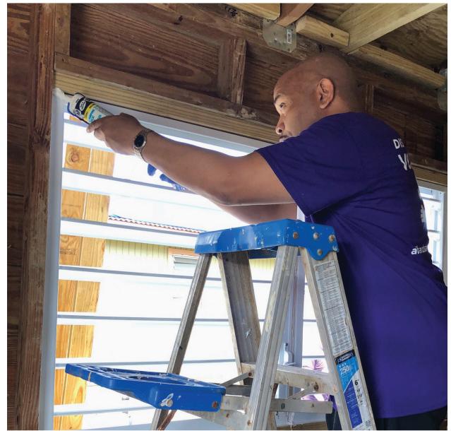
Assemblyman Heastie helps repair damage from the hurricanes in the Virgin Islands.
