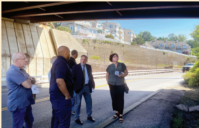
Viewing deterioration under the High Street Bridge in Dobbs Ferry
